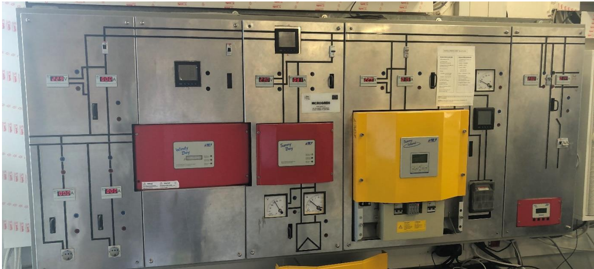
Figure 4: Low-voltage microgrid in the host lab.
