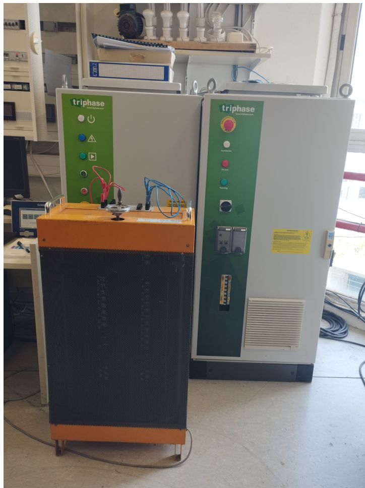
Figure 3: Triphase 15kV configurable power converter operated as single phase inverter connected to a resistive load bank.
